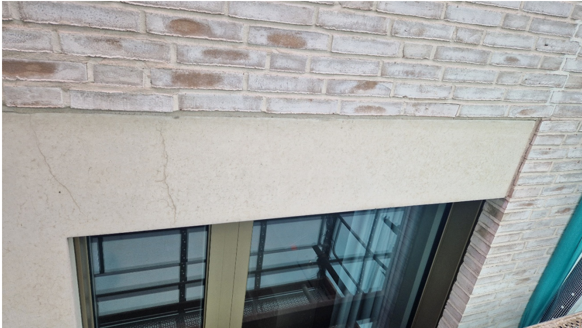
Figure 7: Detail of a composite veneer wall in the area of a window with shear cracks, likely due to statically indeterminate support. The rising veneer wall was built up directly and should have been separated by a horizontal movement joint.
