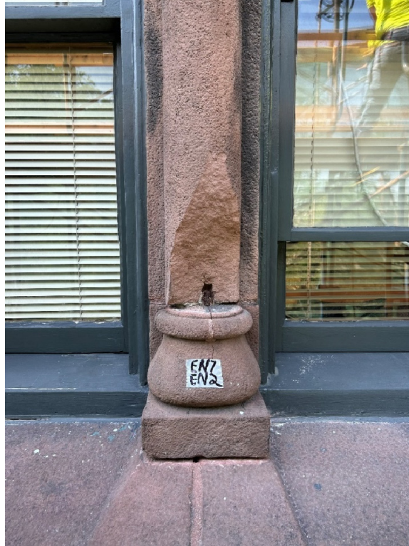
Figure 3: Stone spall in tall, slender stone.
