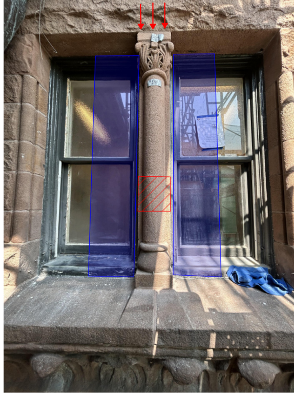
Figure 2: Dutchman repair in slender vertical stone. Red arrows represent gravity loading; blue hatch represents tributary area of wind loading imparted from adjacent windows.
