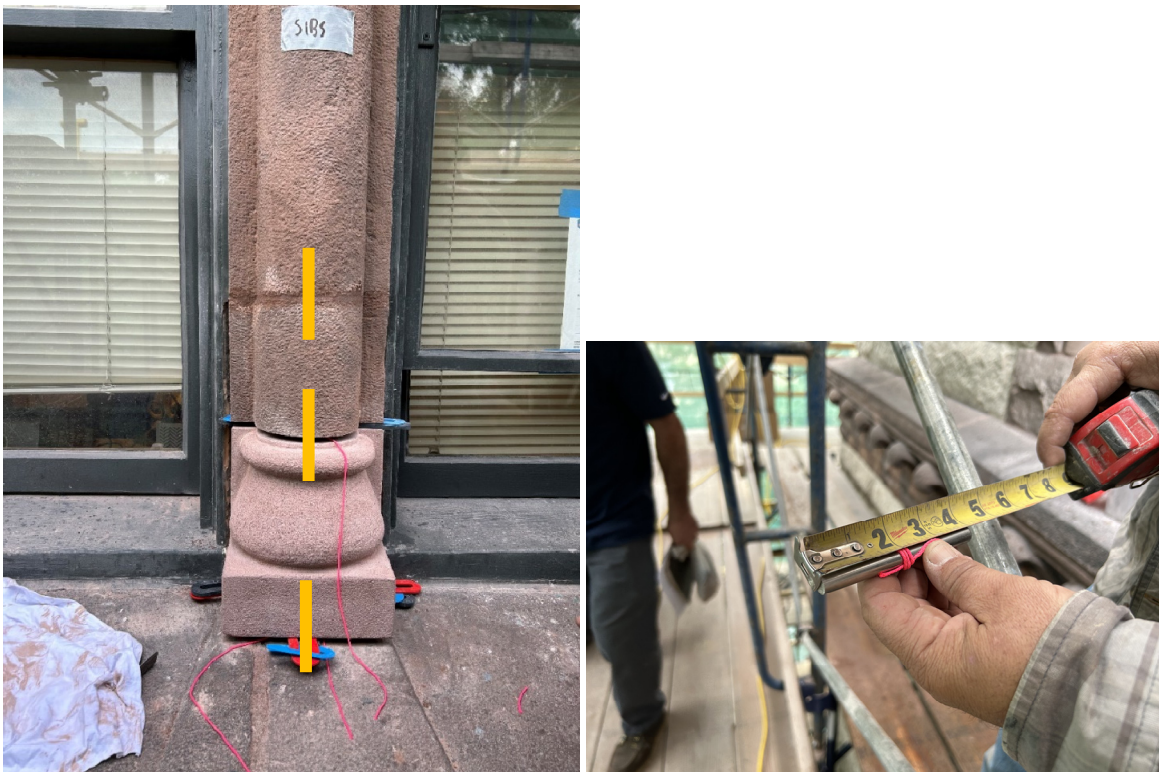
Figure 11: Completed dutchman repair using drop pins. Yellow lines indicate the location of concealed drop pins within the completed repair.
