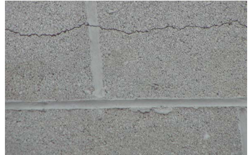
Figure 1. A bond beam with a horizontal crack along its length resulting from placing the grout in freezing temperatures without proper heating and protection.
